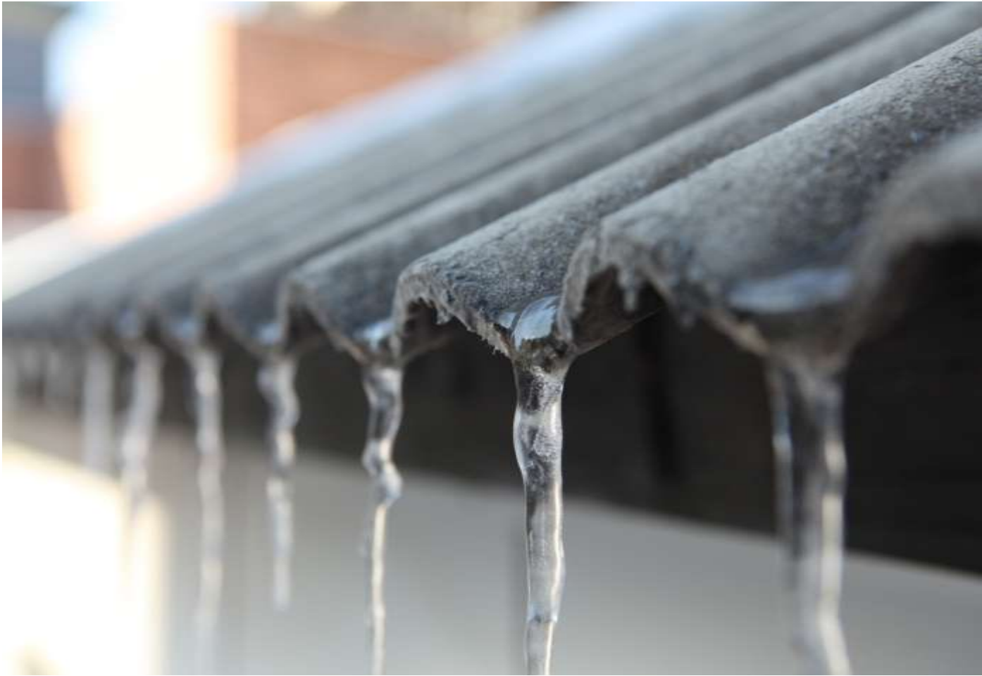
Icicle at slate roof of a school building in Seoul, Korea
