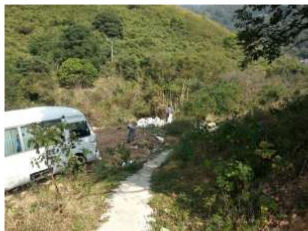
Workers seemed to collect asbestos without any PPE
